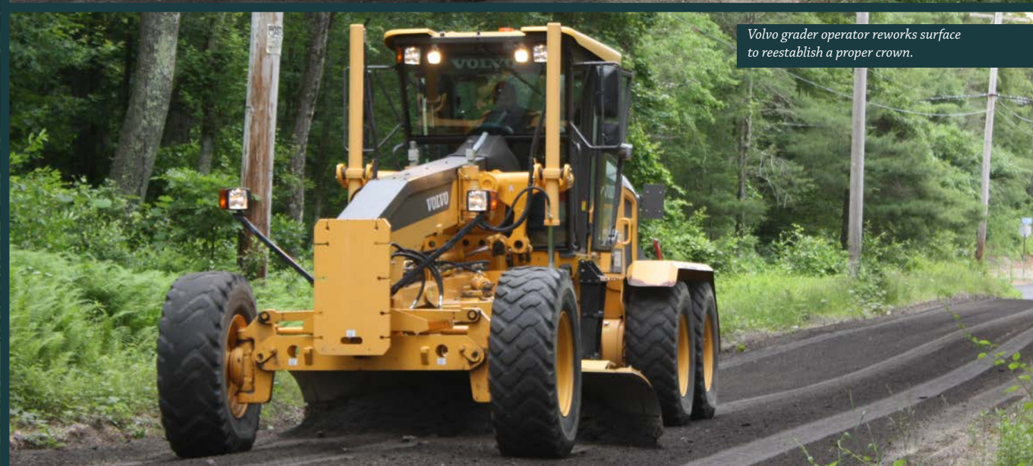
A Mack truck distributor applies Safe Road Services' lignosulfonate compound made from lignin, a byproduct of the paper pulp making process. (Photo courtesy of MEDIABOSS)
